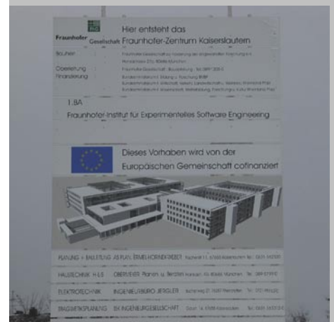
Kick-off: Construction on the third Fraunhofer Center in Germany officially started on 27 October 2003.
